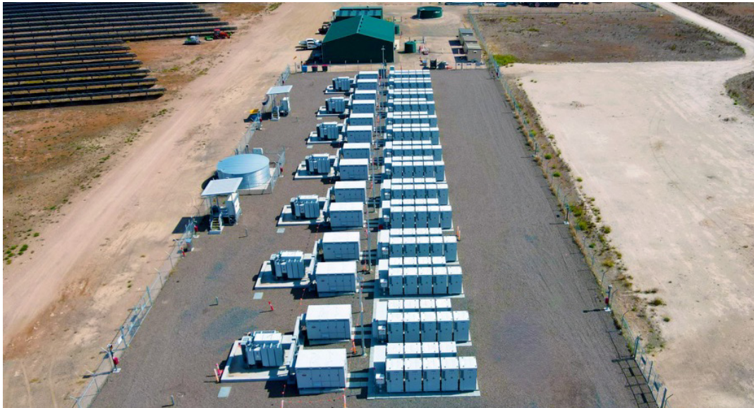
Figure 2 - Tailem Bend II Hybrid BESS, South Australia
