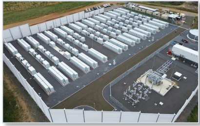
Doosan GridTech chosen to install Neoen's Capital BESS
