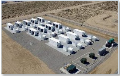
Doosan GridTech chosen to install LADWP's first ESS
